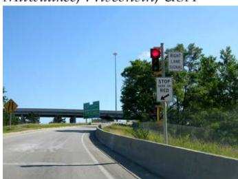
Ramp meter on ramp from Miller Park Way to Interstate 94 east in Milwaukee, Wisconsin, USA
